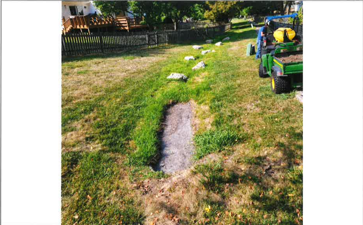
Upstream channel behind SW Marline Dr homes, just downstream of culvert outfall
