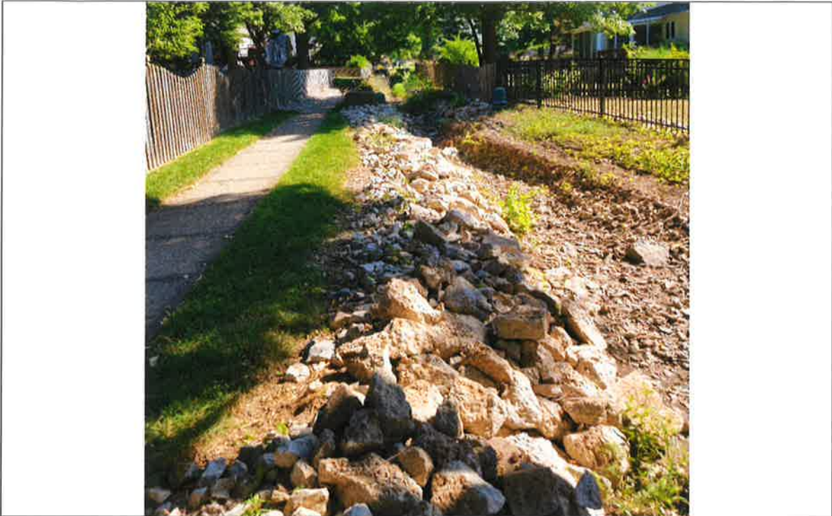
Downstream channel, looking upstream; displaced riprap
