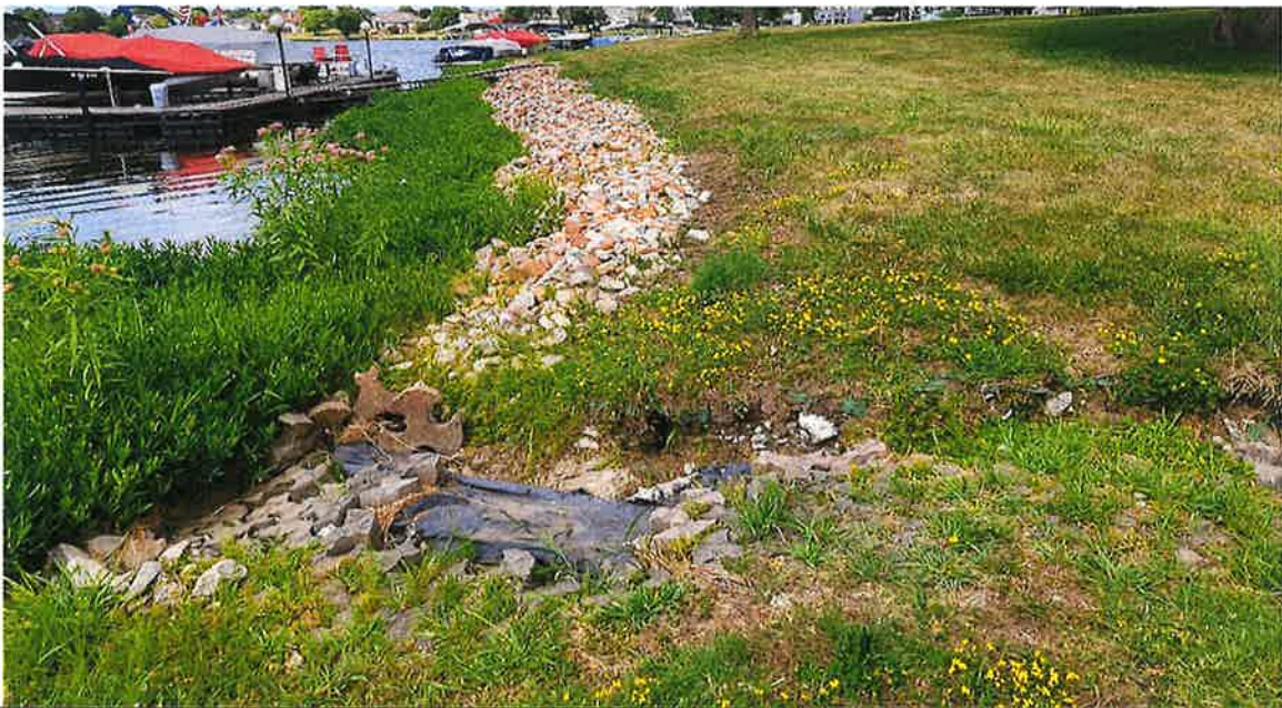
Failure of interlocking blocks in downstream channel
