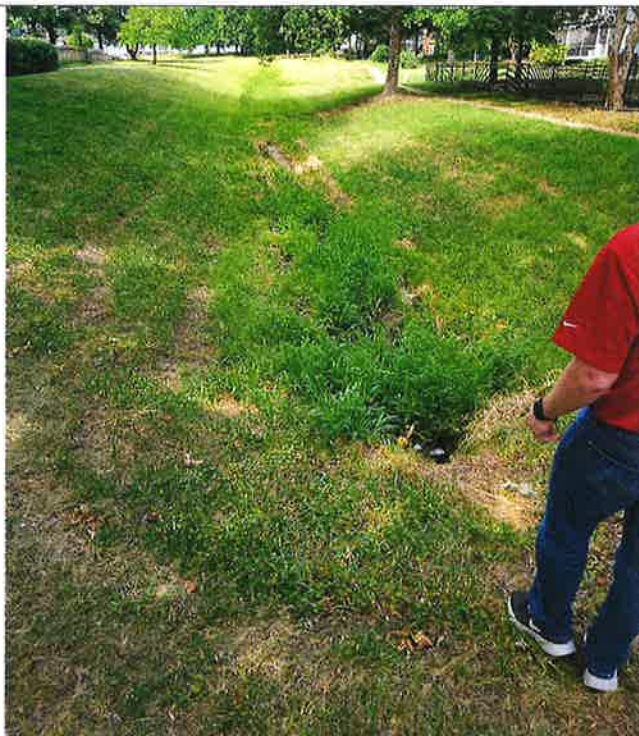
Siltation at upstream culvert outfall
