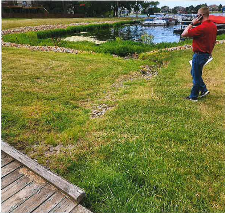
Failure of interlocking blocks in downstream channel
