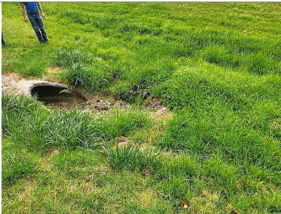
Minor scour at lateral culvert outfall
